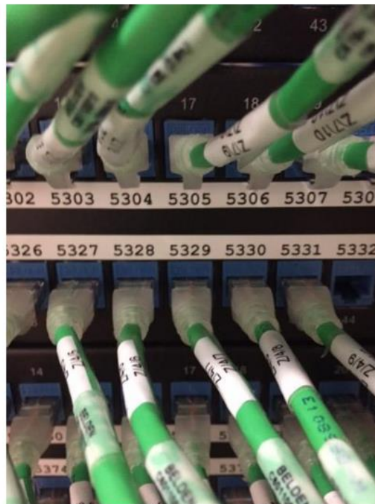
Exhibit 5a: Picture of Patch Panel Labeling
